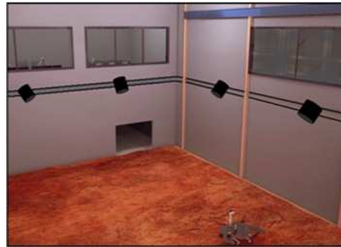
Fig. 8: Positioning cameras located on walls
