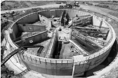
Fig. 2. The SRT antenna basement. The anular structure is 40 m wide and 5 m deep, and will support the 3000-ton antenna.
